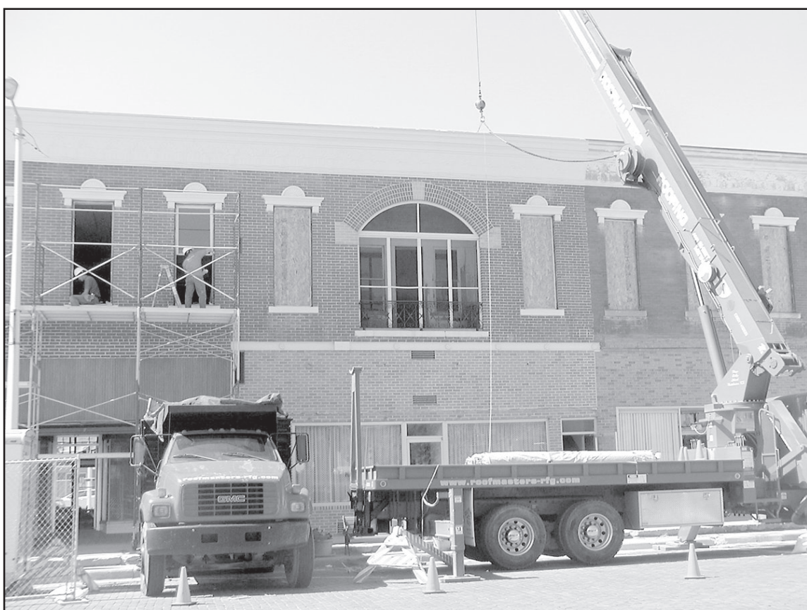
Brian Luther, subcontractor for Schamber Historic Preservation, and Schamber employee Dave Turnbull are seen working on the windows of the east side of the Heaton Building. The project started in August of 2011 and the first phase of the job is coming to an end. This job has provided a lot of business to local merchants, several jobs for area contractors and will provide a beautifully restored building for the new owners once it is completed.
