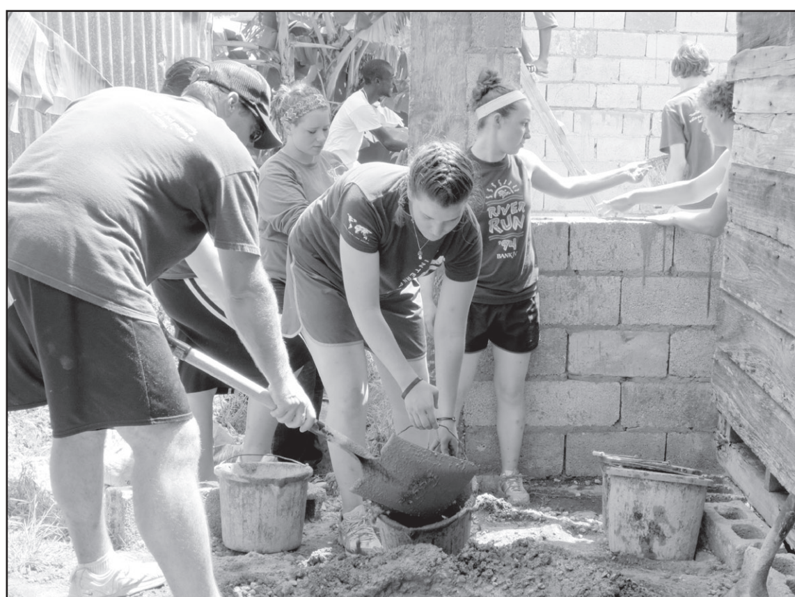
Teens for Christ youth help to build a home on their mission trip. In the front are Kiersten Klinger of Phillipsburg, Laura Thompson of Hutchinson, Heather Harshbarger of Ingalls, in the back ground. In the house are Jude Wallinger and Caleb Koerperich from Oberlin. The gentleman in the front shoveling the concrete into the bucket is the Executive Director Brian Fischer.
