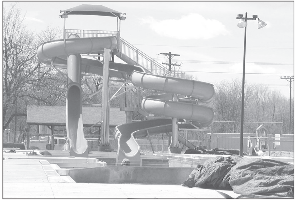
Progress is coming along on the new swimming pool being built in Norton. The construction crew has both new slides put into place along with the pool house. Now for the rest of the pool to be completed so the water can flow!
