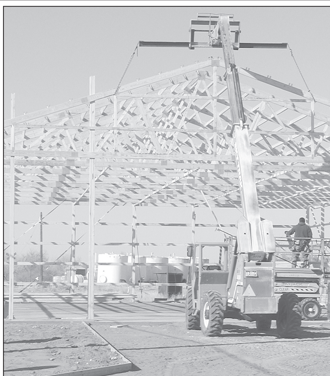
SHED RAISING — The new St. Francis Equity Feed store building is quickly going up on River and Jackson streets. Herald staff photo by Karen Krien
