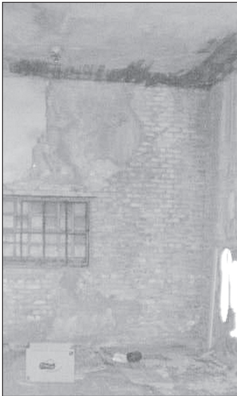
DETERIORATION is evident in the northeast corner of the backroom in the band shell. Much of the money raised will go to renovate these areas.
