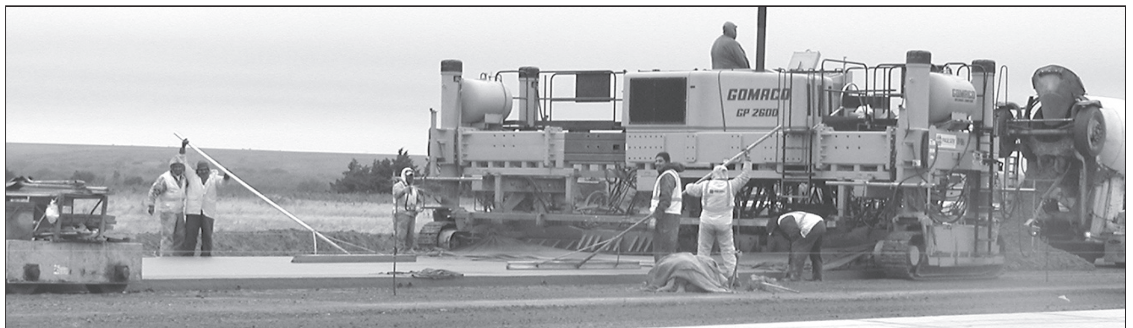
NEITHER COLD OR DAMP kept workers from pouring the concrete for the new runway at the airport Monday. The runway could be open by the first of November.
