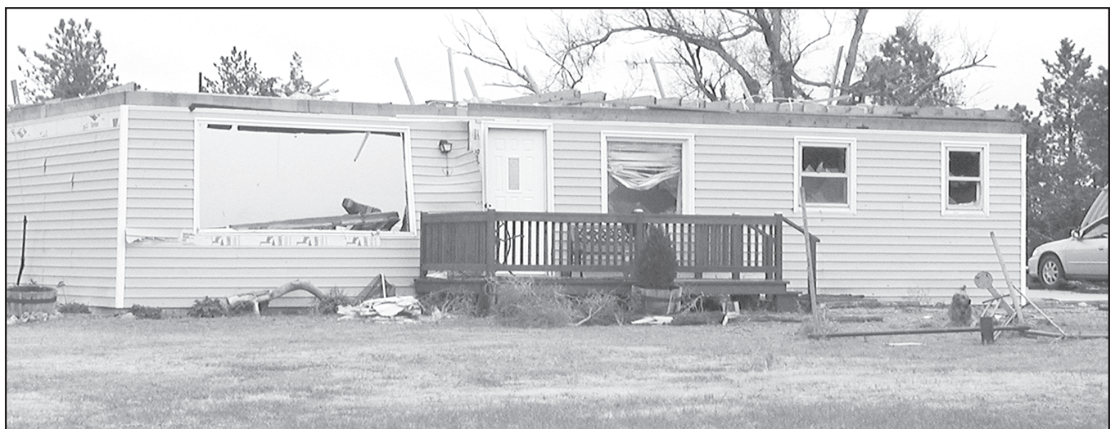
John and Maria Kamla home with the roof ripped off Photo by Melinda Basnett
