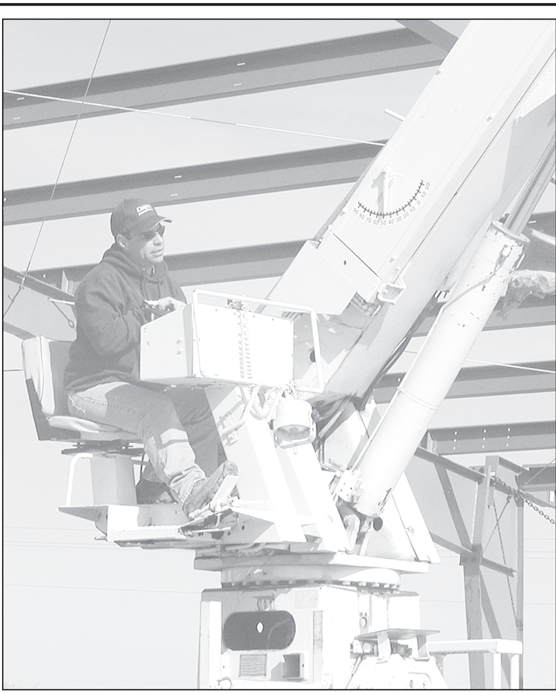
JR LANDEMBERGER maneuvers the overhead beams into place at the new emergency building. Herald staff photo by Casey McCormick
