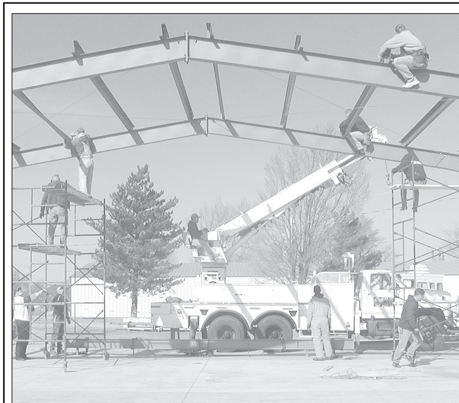
VOLUNTEERS gathered to work on the new emergency building Saturday. The building is being put up with a KAN STEP grant funding the materials but it will take volunteer manpower to complete the job. The building is to be completed by March.
