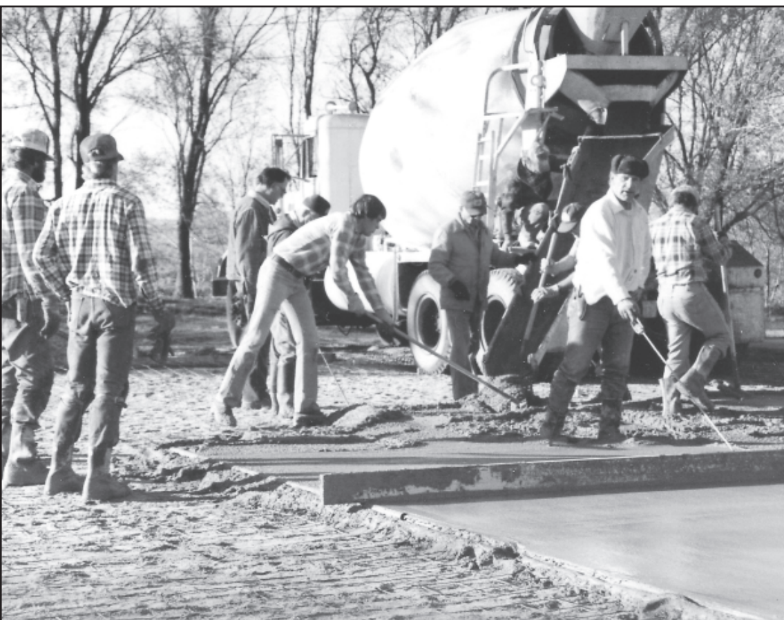
VOLUNTEERS gathered to begin the construction of the new museum. An open house is set to commemorate the history from when the museum was established.
