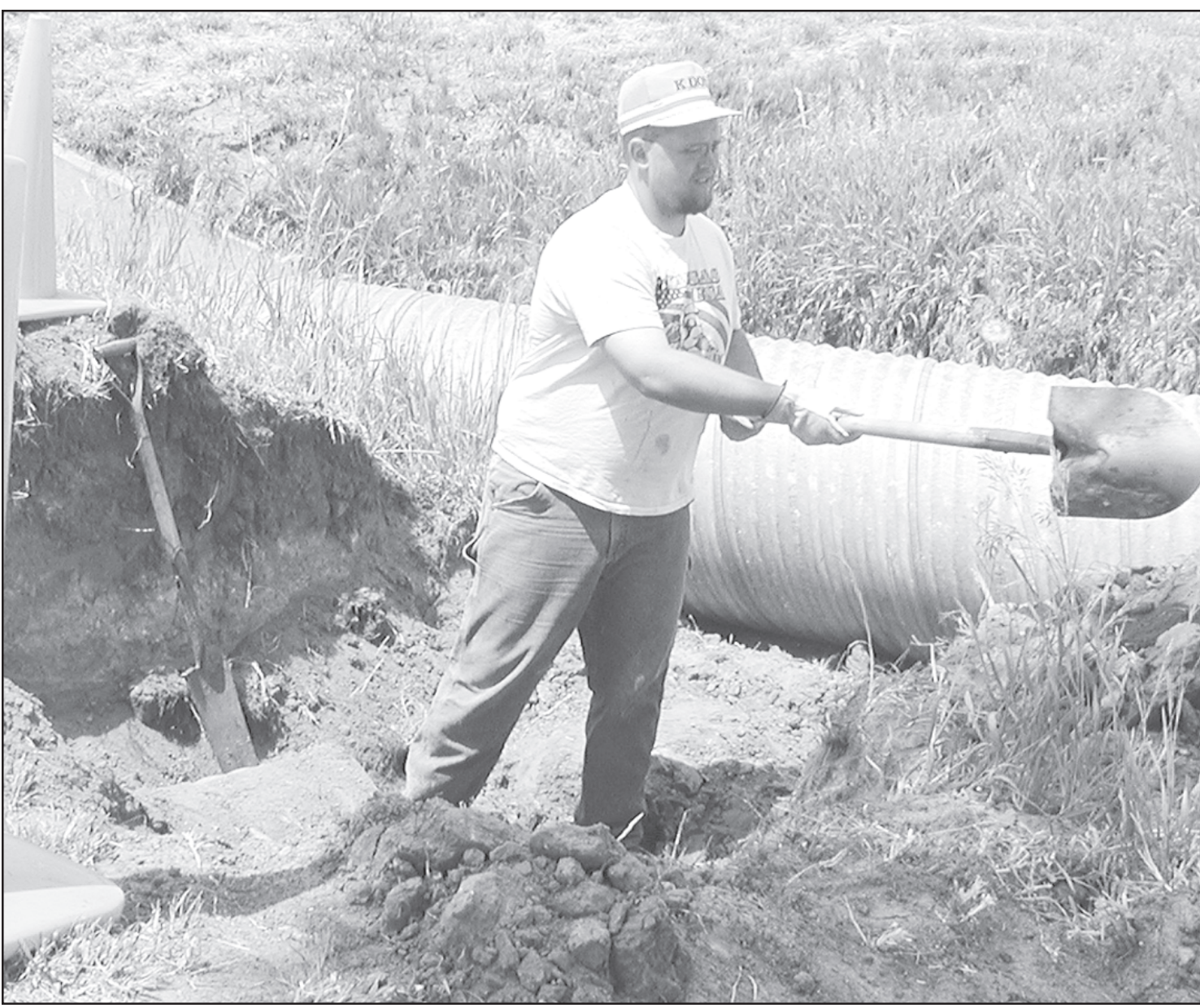
SETH SWIHART is putting in a culvert north of the state building in St. Francis.
