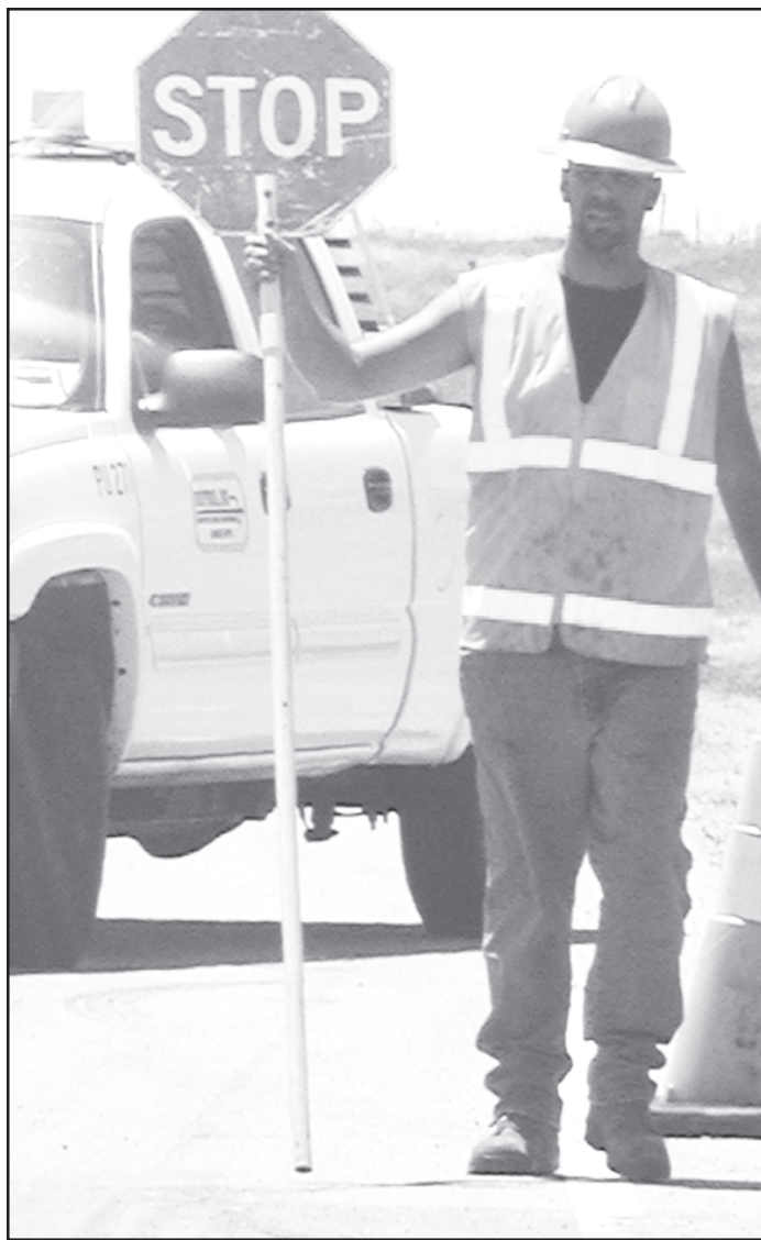
STOPPING TRAFFIC — Curtis Neal, Phoenix, is working for Dustrol Inc. The crew plans to be here only nine or 10 days.
