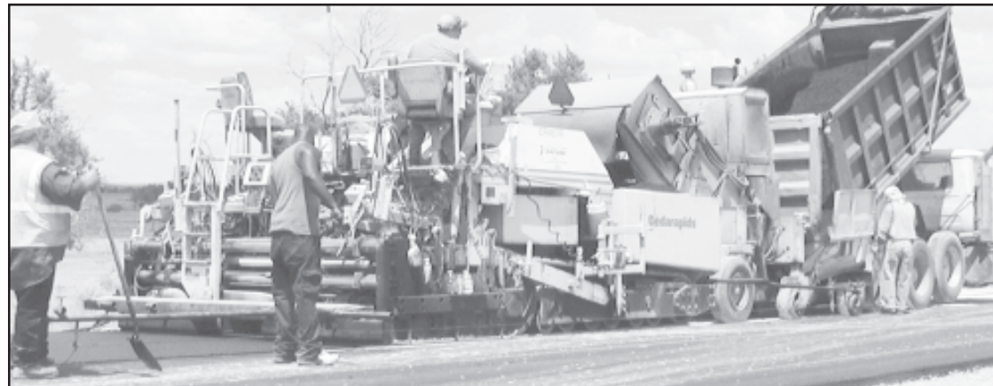
ASPHALT IS TRUCKED to the River Road southwest of St. Francis, then dumped into the machine that lays down the asphalt. It was a hot job on Monday.
