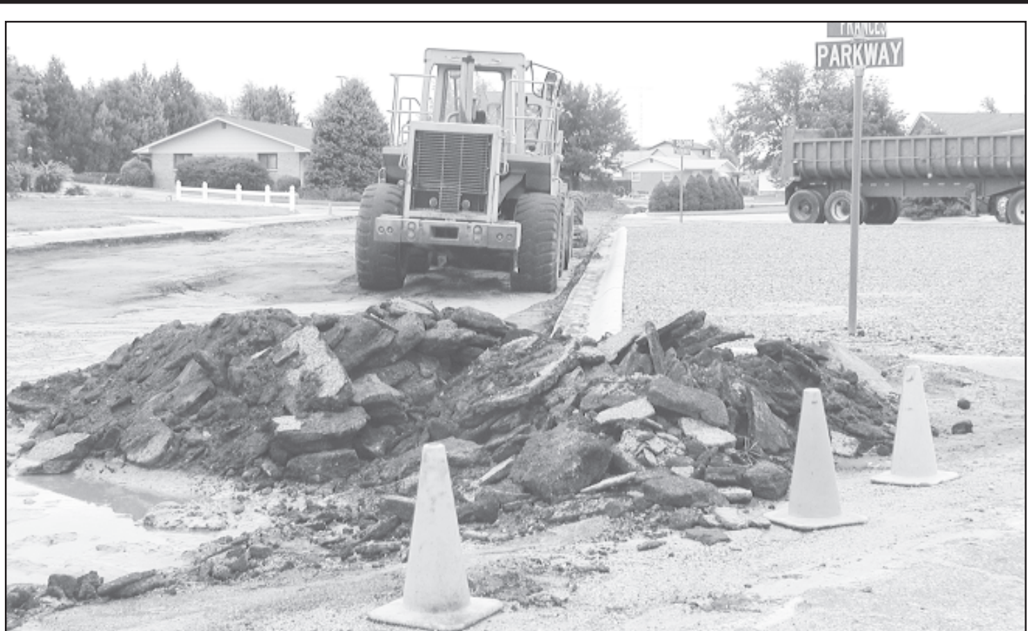
STREET WORK BEGINS on Parkway Drive. The street repairs have been a controversial matter with residents and
