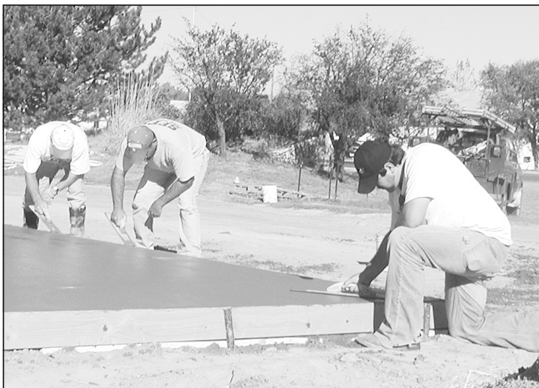
VOLUNTEERS ARE TAKING ADVANTAGE of the warm weather to get the cement on the approaches. In another week, the roof will go on. City Council At the Oct. 2 meeting, the St. Francis City Council was told that the roof on the emergency building would be put on the weekend of Oct. 13 and 14.
