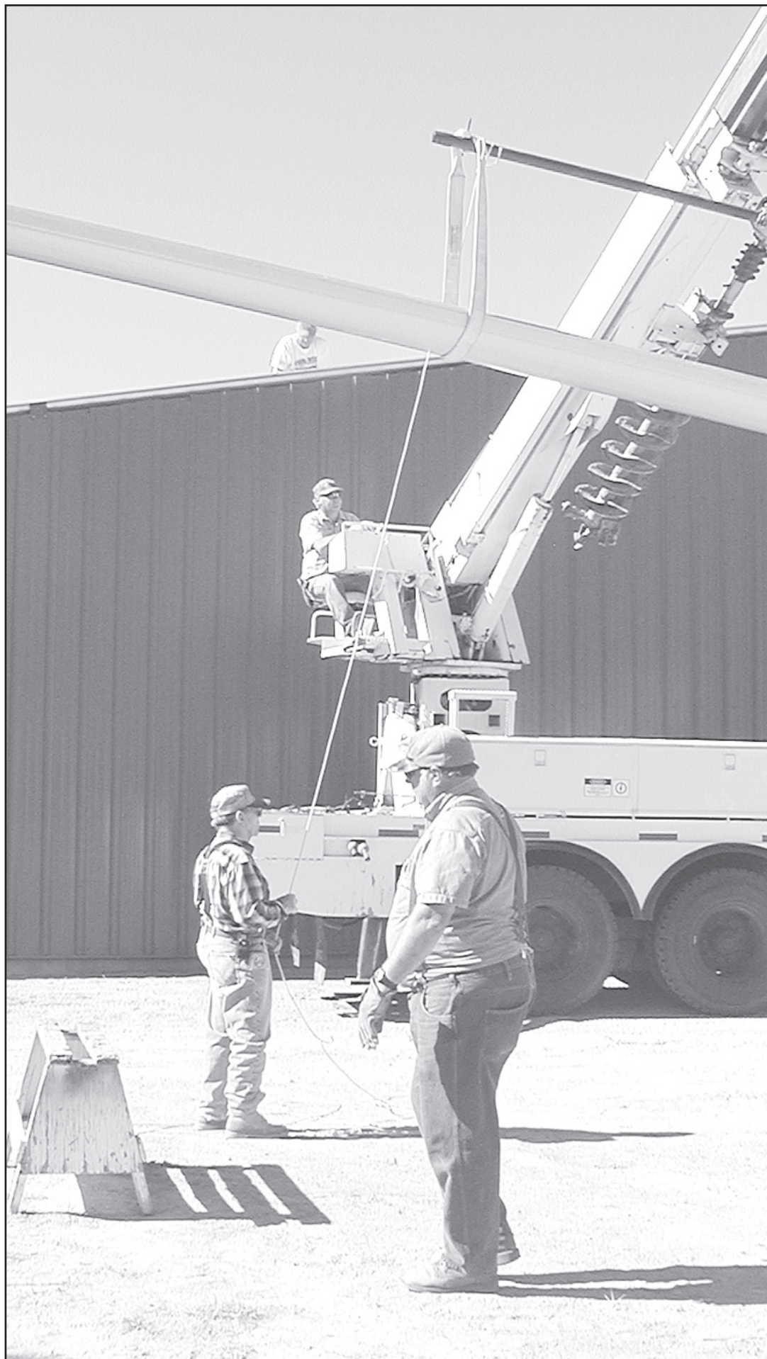
WORK ON THE EMERGENCY building is very noticeable these days. Volunteers have been busy for over a week and do not plan to stop until the roof is on. When cold weather set in, work will begin on the inside and more volunteers will be needed. Everyone should stop by and see what is going on and how they can help. Herald staff photo by Casey McCormick
