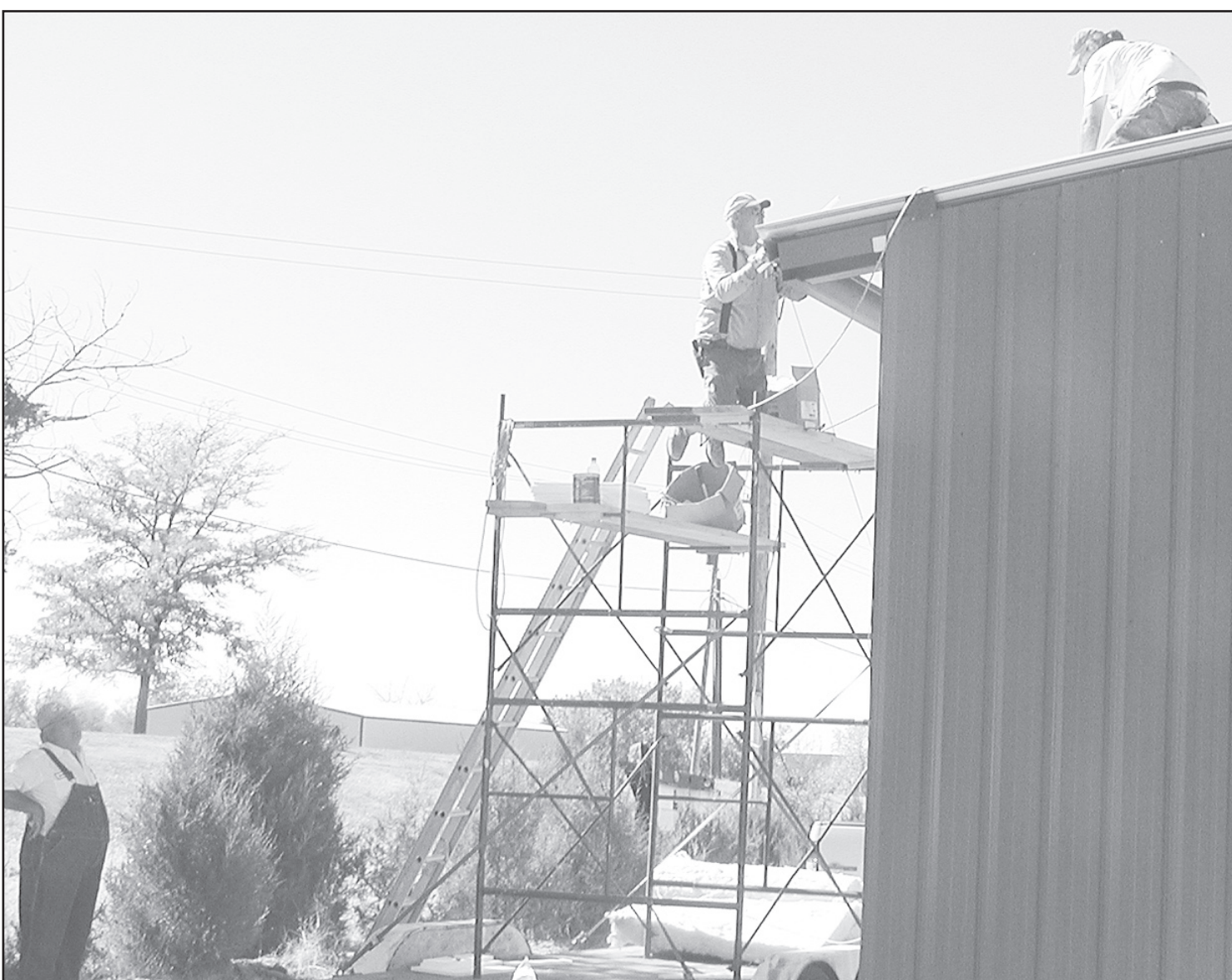
VOLUNTEERS WORKING — Several people have been busy at the new emergency building to get the roof on before the weather gets cold and snowy. Those pictured are Ronnie Krien, Sam Miller and Scott Schultz.
