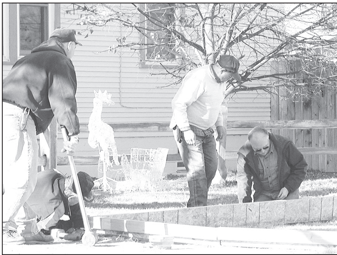
ICE SKATING RINK is once again being installed at the Steve and Connie Jenkins' home. Doing the work (l to r) Roger Orth, Milton Lampe, Dale Patton and Tony Howard.
