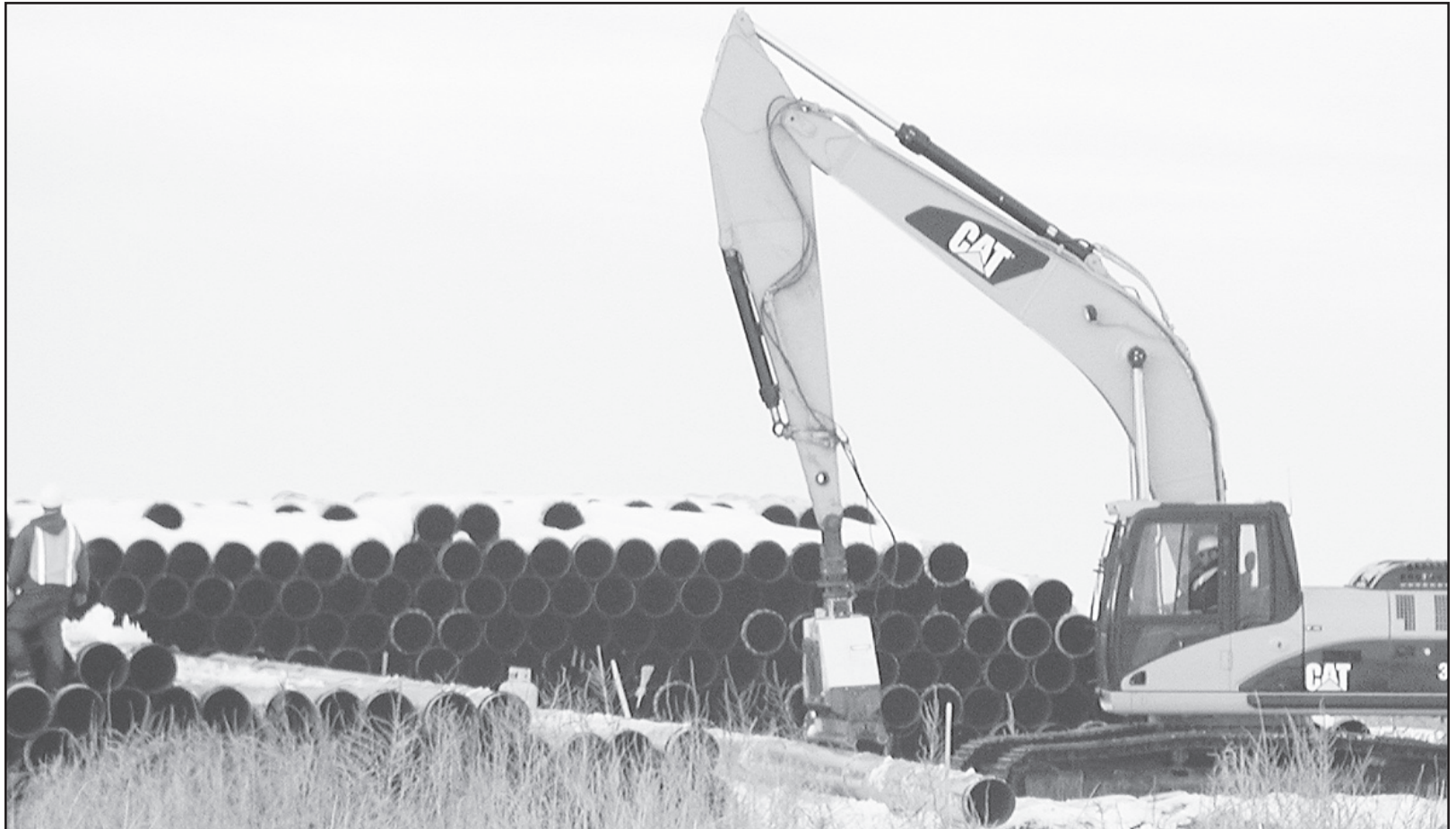
OVERLAND PASS CREW is removing pipe stored northwest of Bird City and loading it onto nearby trucks to be transported to work site. Construction is scheduled to be completed early this year. Times staff photo by Linda Schneider
