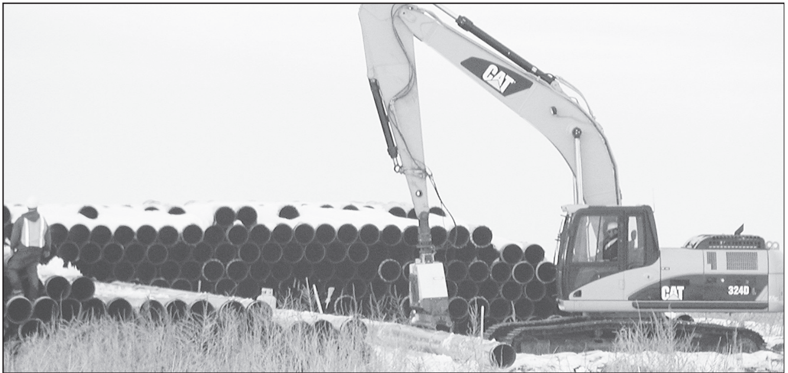
ROWS OF GREEN PIPE are moving as the new line goes through Cheyenne County. The pipes have been piled near the railroad track in Bird City.
