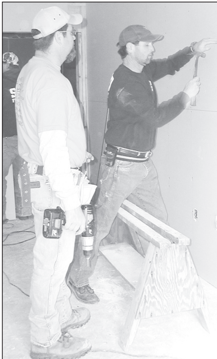
STEVE JENKINS and other work on the new emergency building. Deadline is March 15.
