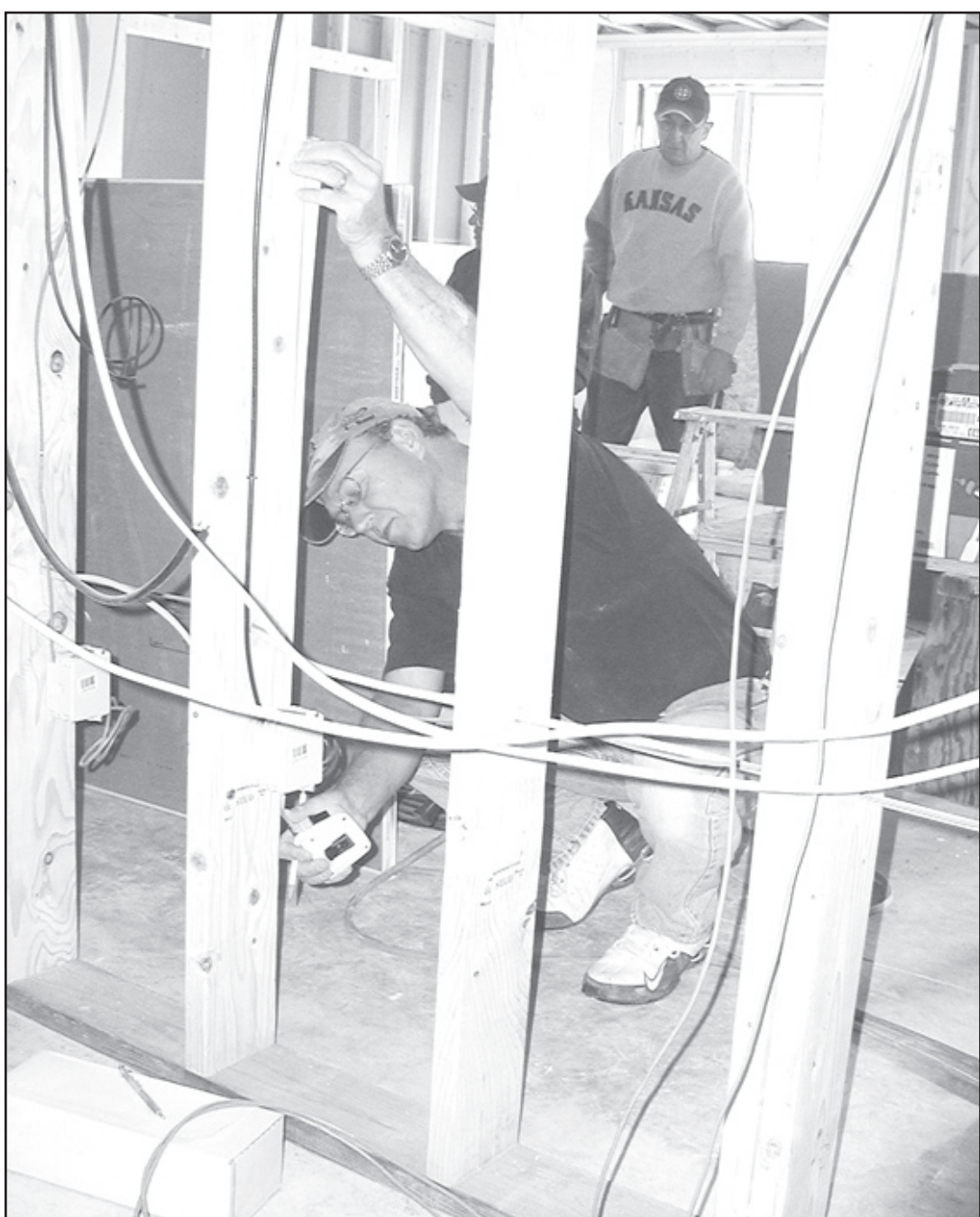
VOLUNTEERS WERE HARD AT WORK at the St. Francis Emergency Service building on Saturday. Kelly Frewen, fireman, is putting in an electrical outlet. The building must be finished by March 15 to comply with the grant.
