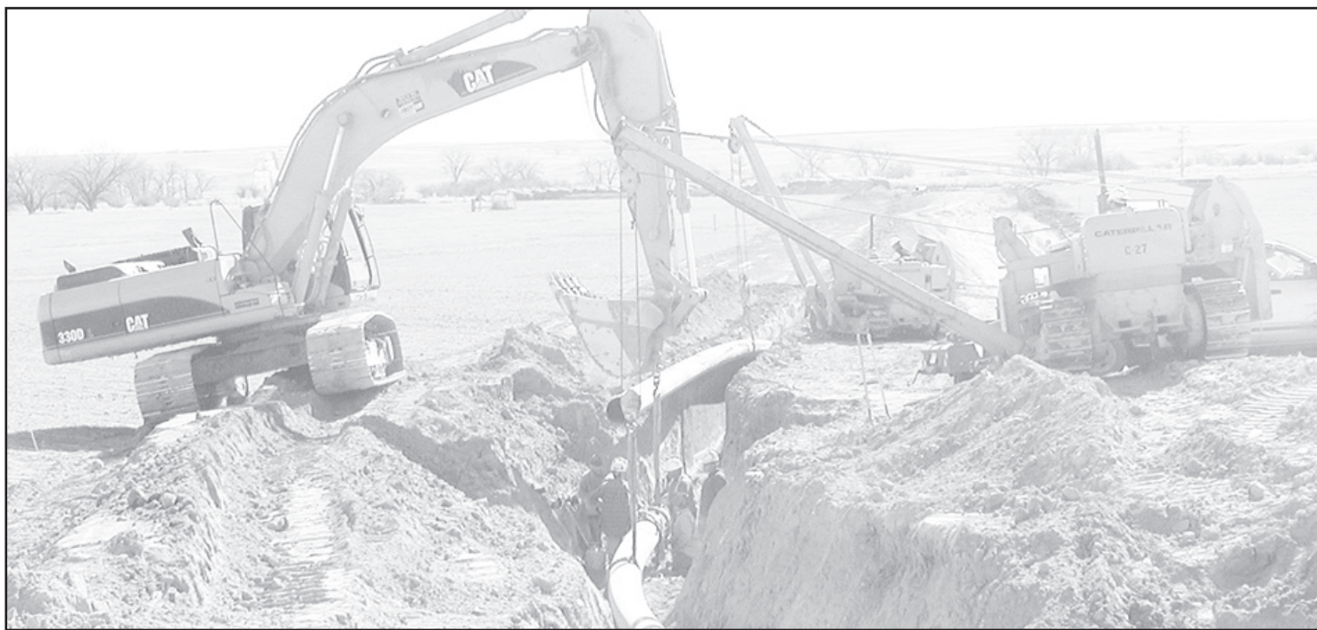
LOWERING 20-FOOT SECTION of steel pipe to carry natural gas — the pipe is being laid across Cheyenne County. This pipe is being put in out north of St. Francis.
