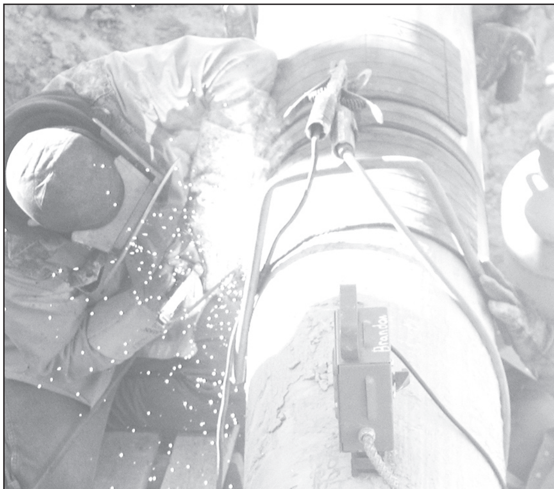
WELDER JOINS PIPES — one of the many steps to laying the pipe for the Overland Pass Pipeline.
