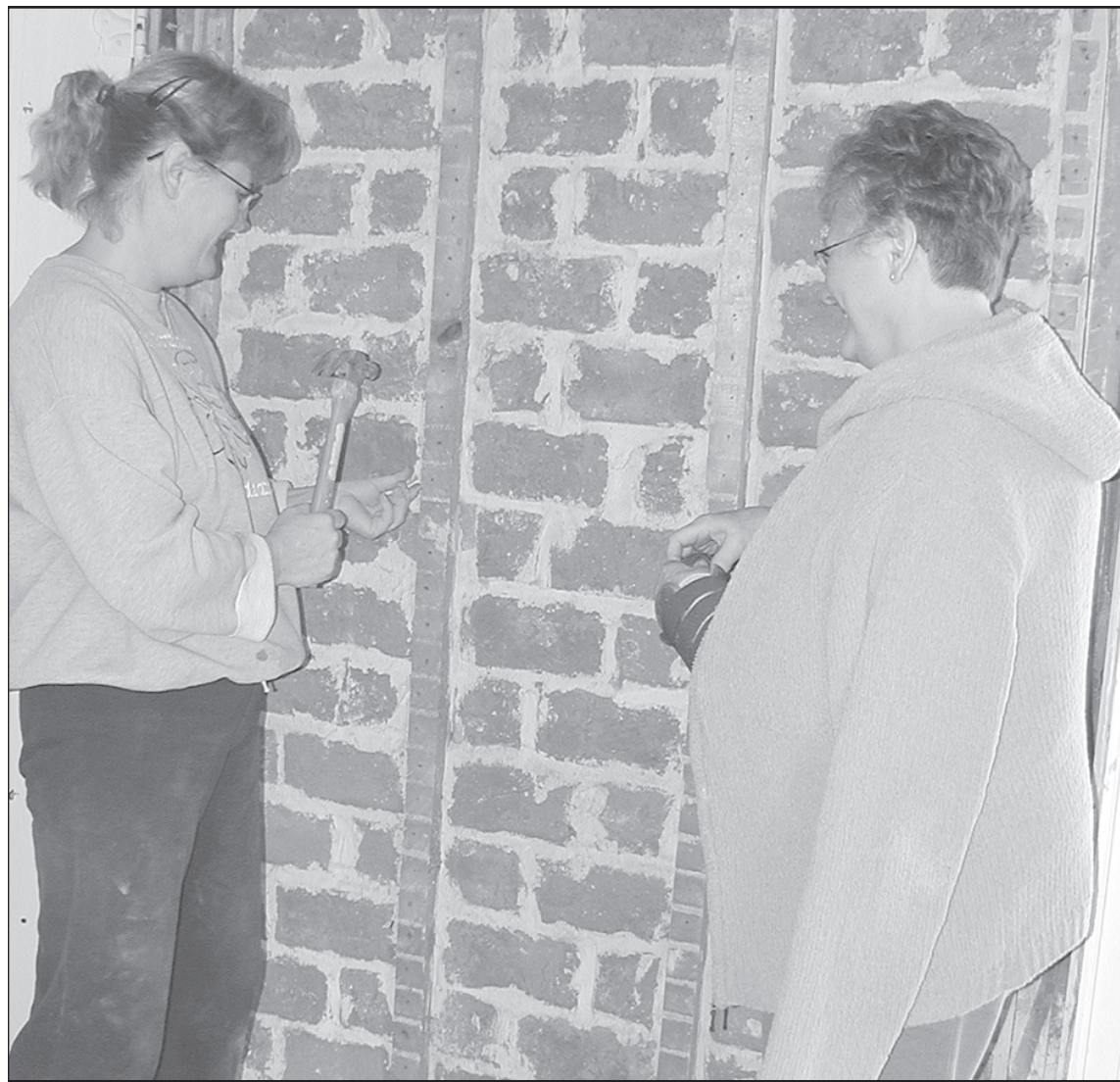
SOD BLOCKS were found under the plaster and lath when Esther Confer, right, and her daughter, Tammi Sherlock, remodeled the 1889 house. Herald staff photo by Karen Krien
