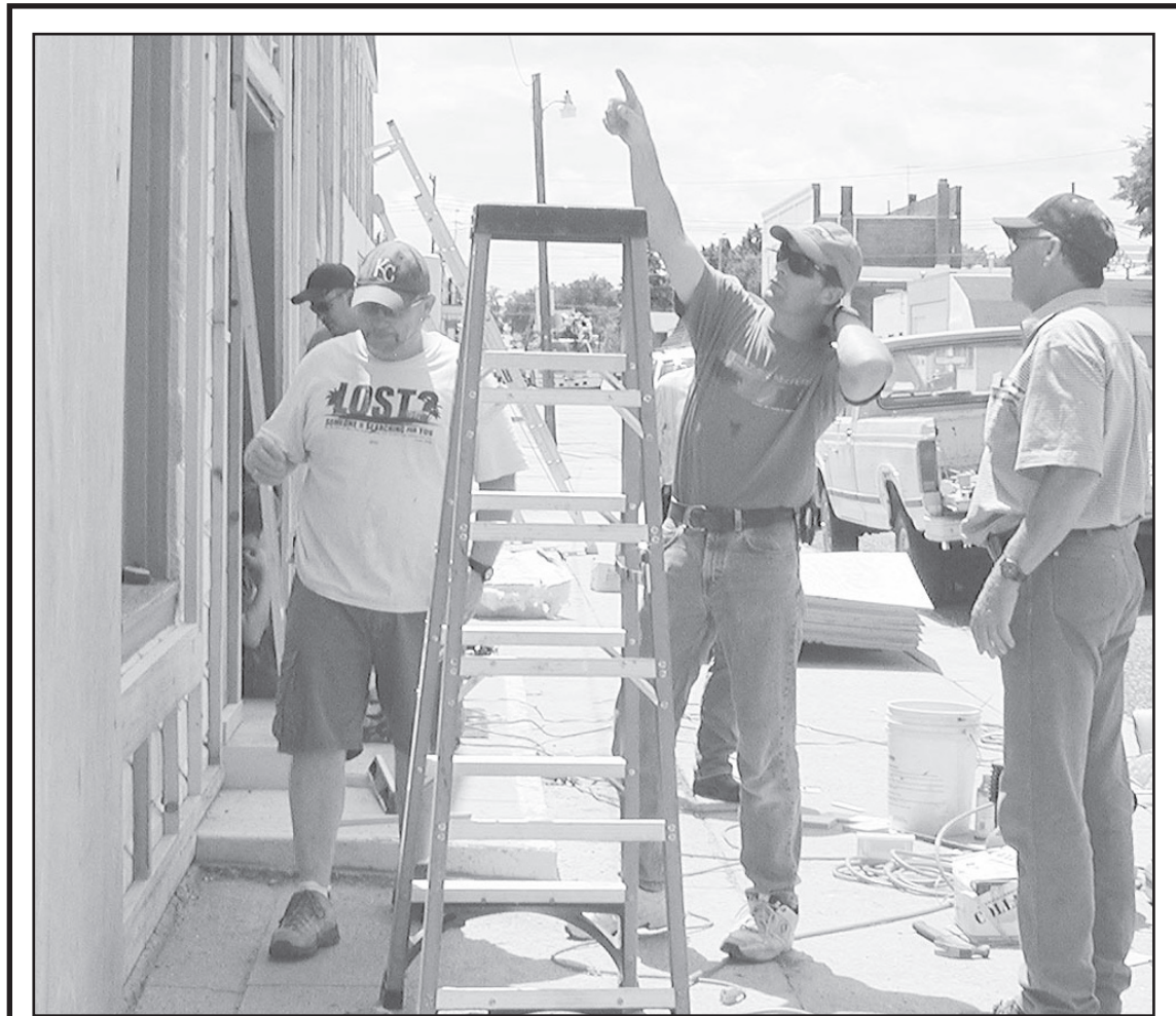
ST. FRANCIS Community Church get a new look. Kary Zweygardt, Tim Schmid and Rodney Shay work to reface the church.
