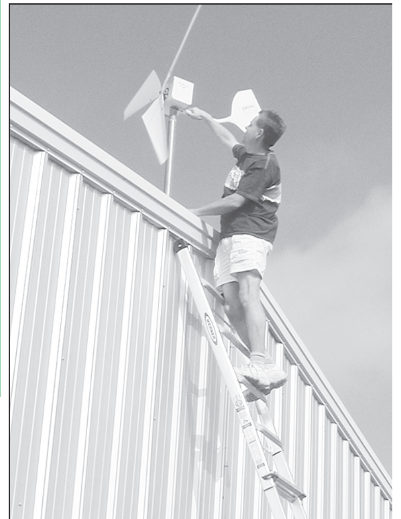
MARLIN QUEEN climbs the ladder to adjust the wind turbine at the Reeser building. He, along with Ron Wieck and Tanner and Ben Lacy installed the wind power equipment.
