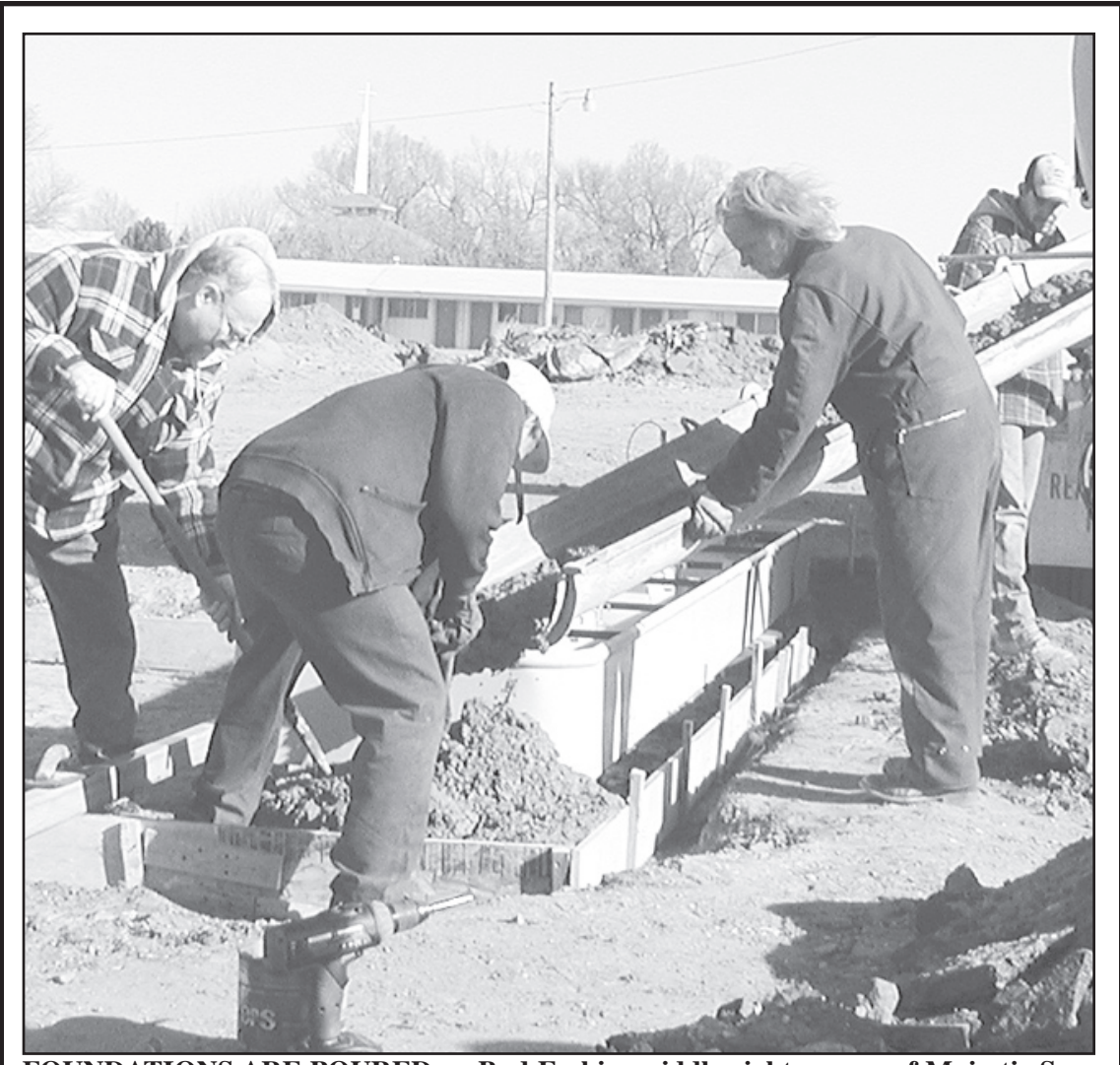
FOUNDATIONS ARE POURED — Bud Erskin, middle right, owner of Majestic Service on U.S. 36, is getting closer to opening his business to sell gas. Part of the pumps are already set and ready to go. Within the week, Mr. Erskin plans to have the rest of them ready.
