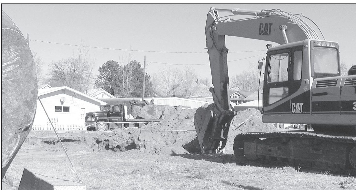
GROUND IS BEING BROKEN for the new Western State Bank building in St. Francis. The new bank will be located at the corner of Washington and Francis Streets
