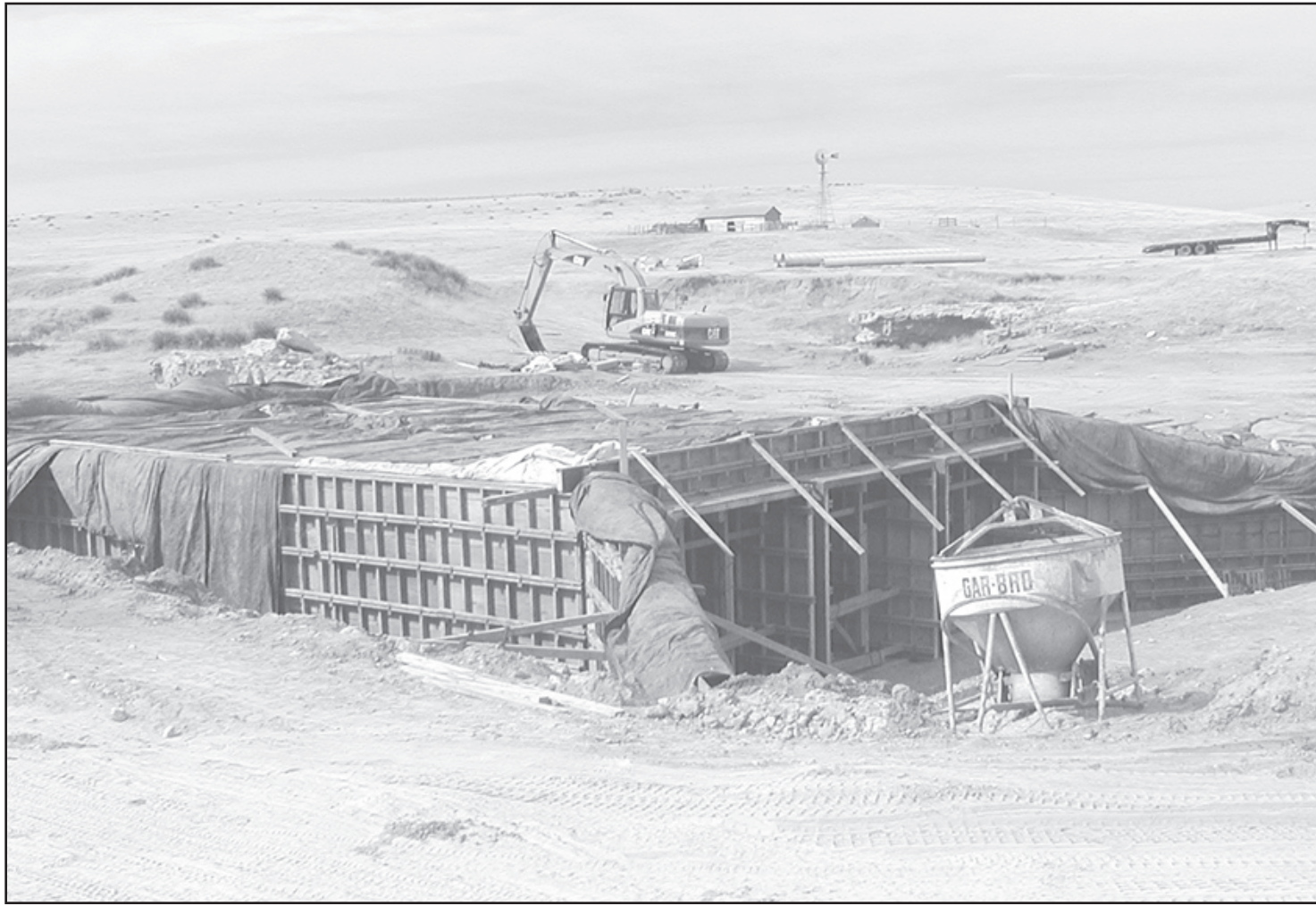
CONSTRUCTION IS NOW TAKING PLACE at the Runzel Bridge, west of St. Francis.
