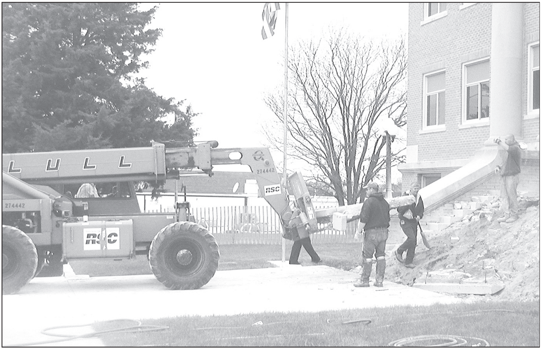
COURTHOUSE STEPS in St. Francis are being demolished and the new steps will soon be going in. Workers began work last Thursday.
