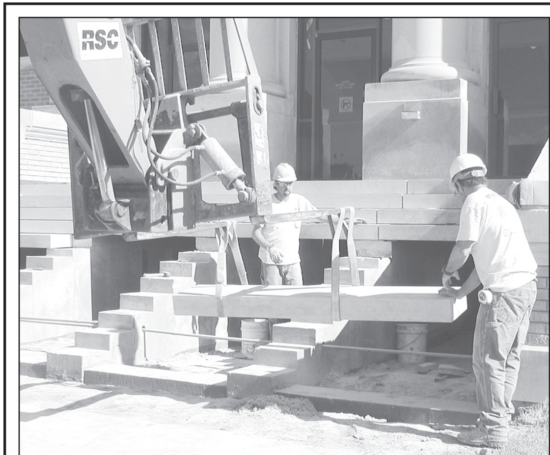
COURTHOUSE STEPS are being put in. Head contractor Cary Stupka, driving the large lift moving the slabs of limestone, left, and his crew have been working whether it is hot or cold in order to get the steps in as quickly as possible. The laying of the stone is a tedious job and pillars have been installed to make sure the stones will stay in place.
