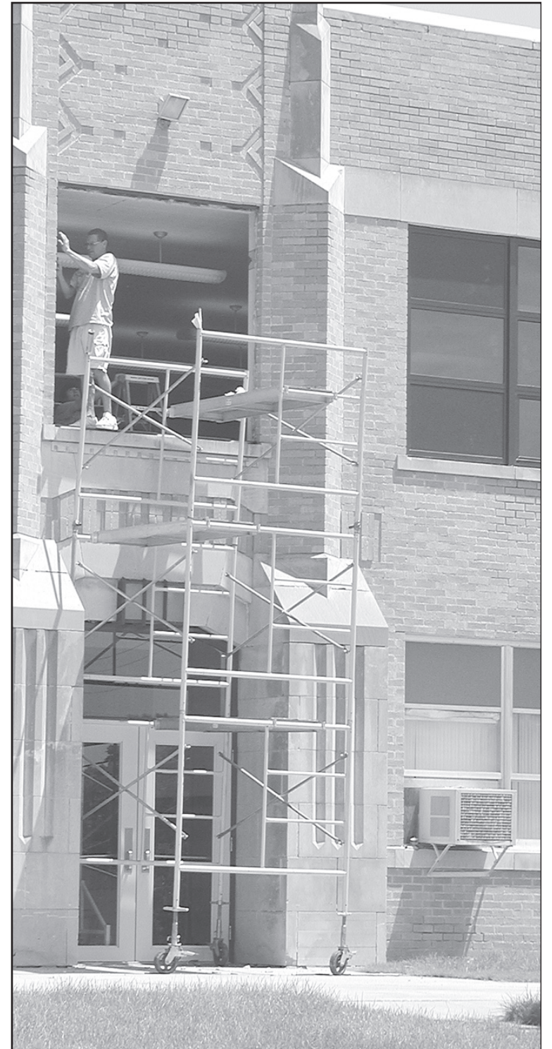
NEW WINDOWS are being installed on the west side of the high school. The new windows on the left have brown frames and are all glass, letting in more light.
