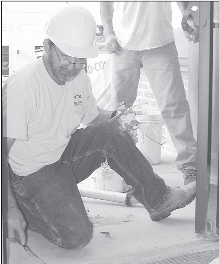
WORKMEN FINISH up the floor beneath the doors at the top of the new steps. The walk-through inspection is scheduled for Tuesday at 11 p.m.
