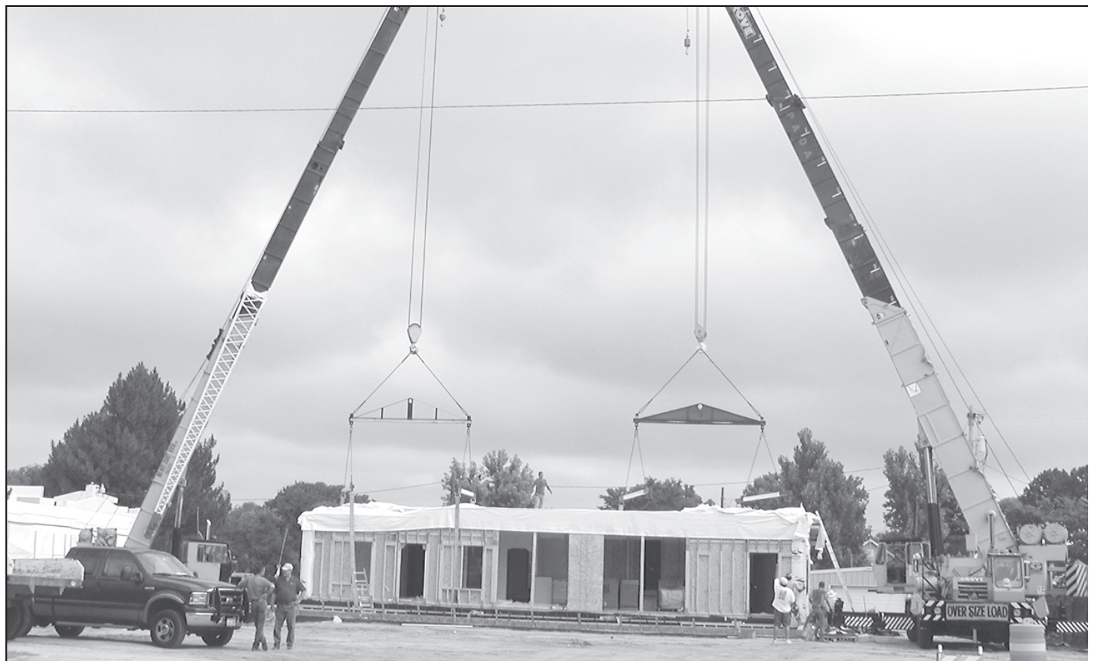
BIG EQUIPMENT lowered the three parts of the new Western State Bank on Thursday. There is much work to be done on the bank before it opens. However, the tentative date is sometime in the fall.
