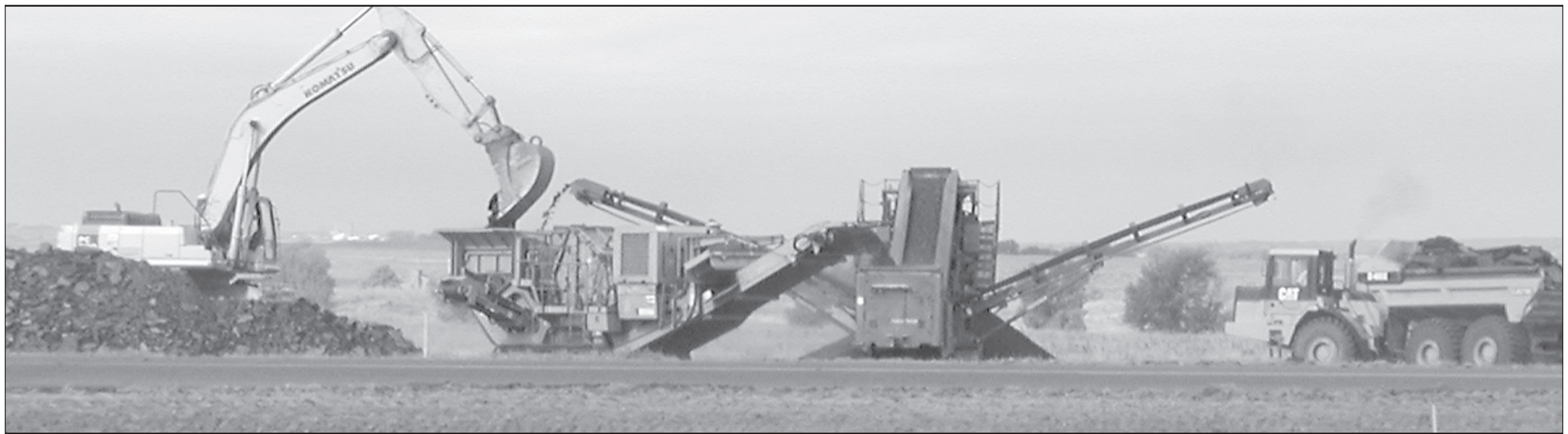
HEAVY EQUIPMENT ROLLED in Monday morning and work has begun on the Cheyenne County Airport runway. The runway will be widened and new lights installed. The next step will be lengthening the end of the runway. The runway is expected to be completed by the end of October. Herald staff photo by Karen Krien
