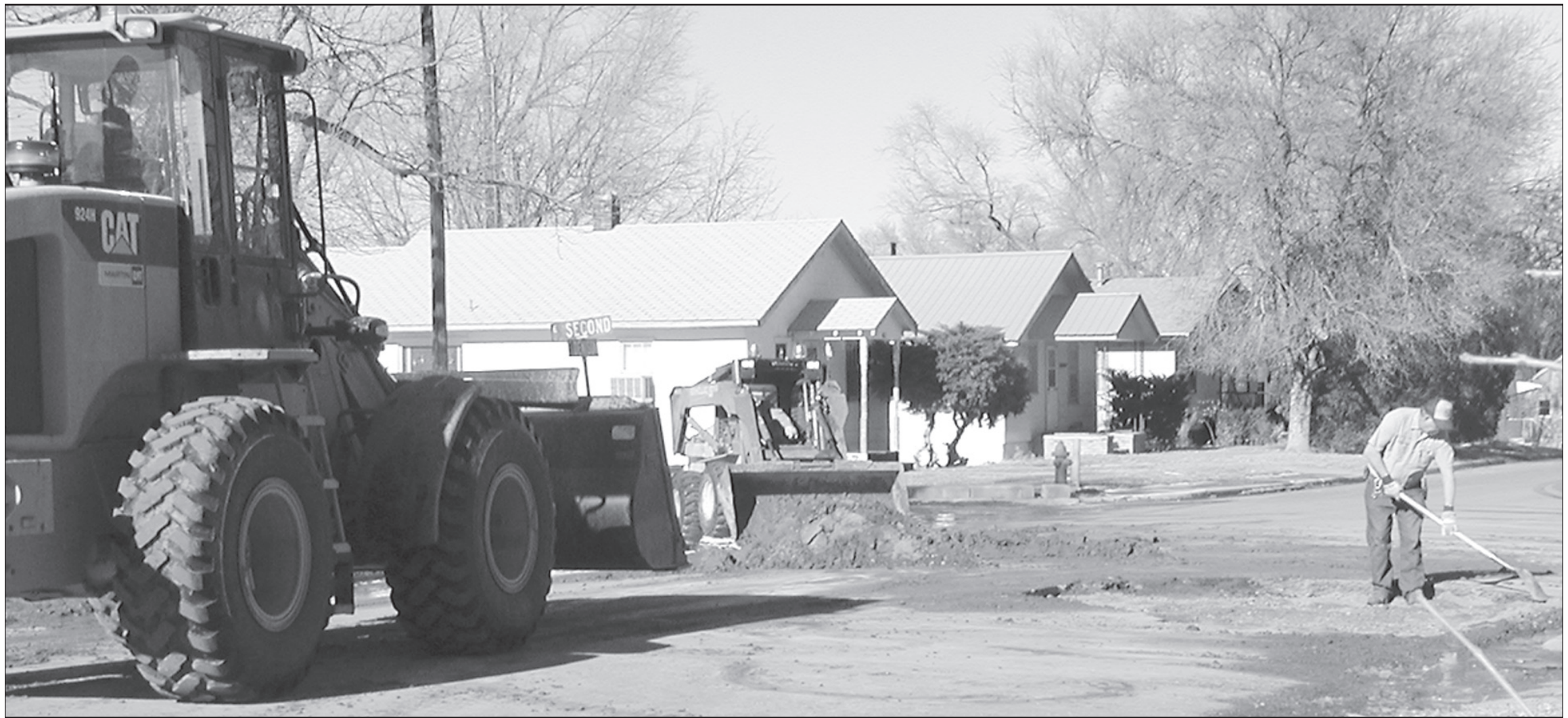
EXTREME TEMPERATURES caused water mains and water meters to freeze during the recent cold spell. St. Francis city crewmen were busy repairing the street on Tuesday after they had dug out a main earlier in the week. With the rake is Earl Hankins.
