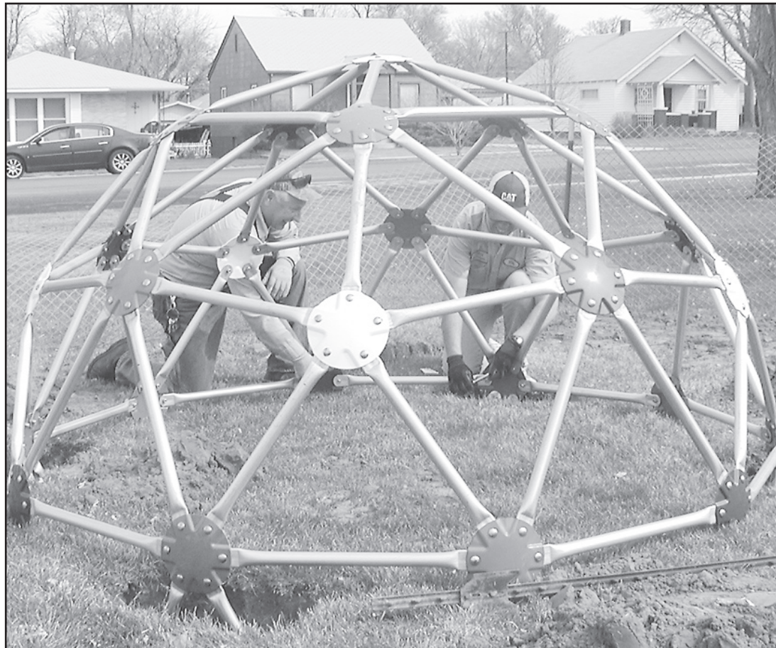
NEW PLAYGROUND EQUIPMENT is being installed in the city park by the city crew. Pictured, left, is Eric Fiala, right, Mike Meyer. The equipment was bought by the St. Francis Area Chamber of Commerce.
