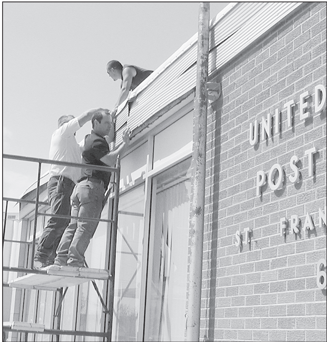
WINDY WEATHER causes damage to the roof at the Post Office. Left to right: Wade Krien; JR Lanenberger, city superintendent; and Nick Chavez work to fasten it down. Herald staff photo by Casey McCormick
