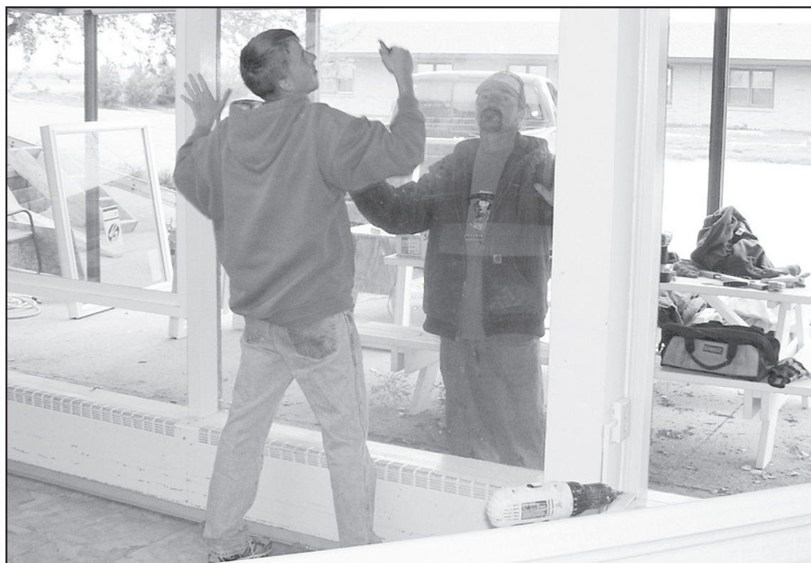
INSTALLING WINDOWS— Andy Horesky (left) and Chad McGovern employees of TJ Improvements put new windows in the Good Samaritan Village dining room.
