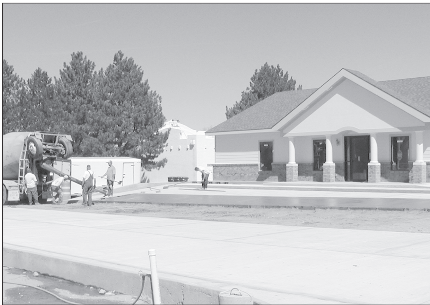
POURING CONCRETE — Work is nearing completion at the new location for Western State Bank in St. Francis. Herald staff photo by Karen Krien
