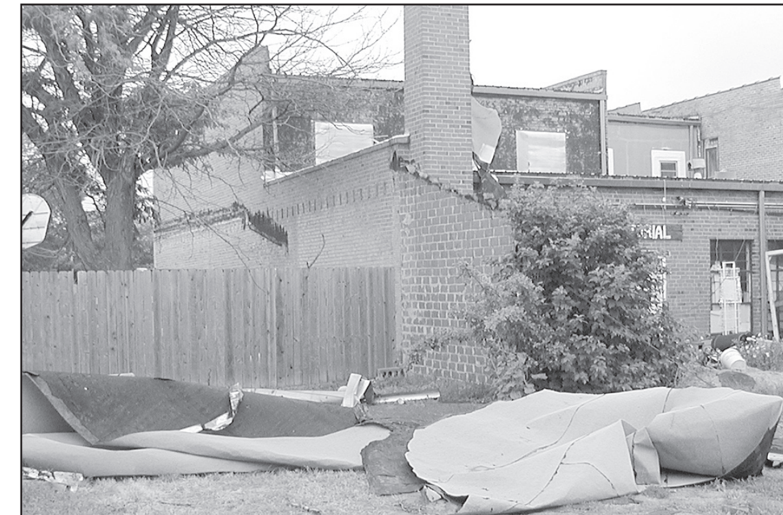
MISSING YOUR ROOF? Zero's is and parts of it were laying in the alley behind the building (above). Right, the wind cleaned the roof right off the building.
