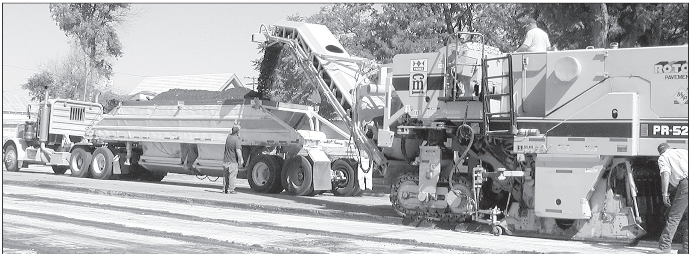
STREETS ON THREE CITY BLOCKS were completely redone this summer. The last one on Jackson Street, above, was work in progress this week. The city superintendent, J.R. Landenberger, said this street would be done after harvest and harvest was pretty much done last week.
