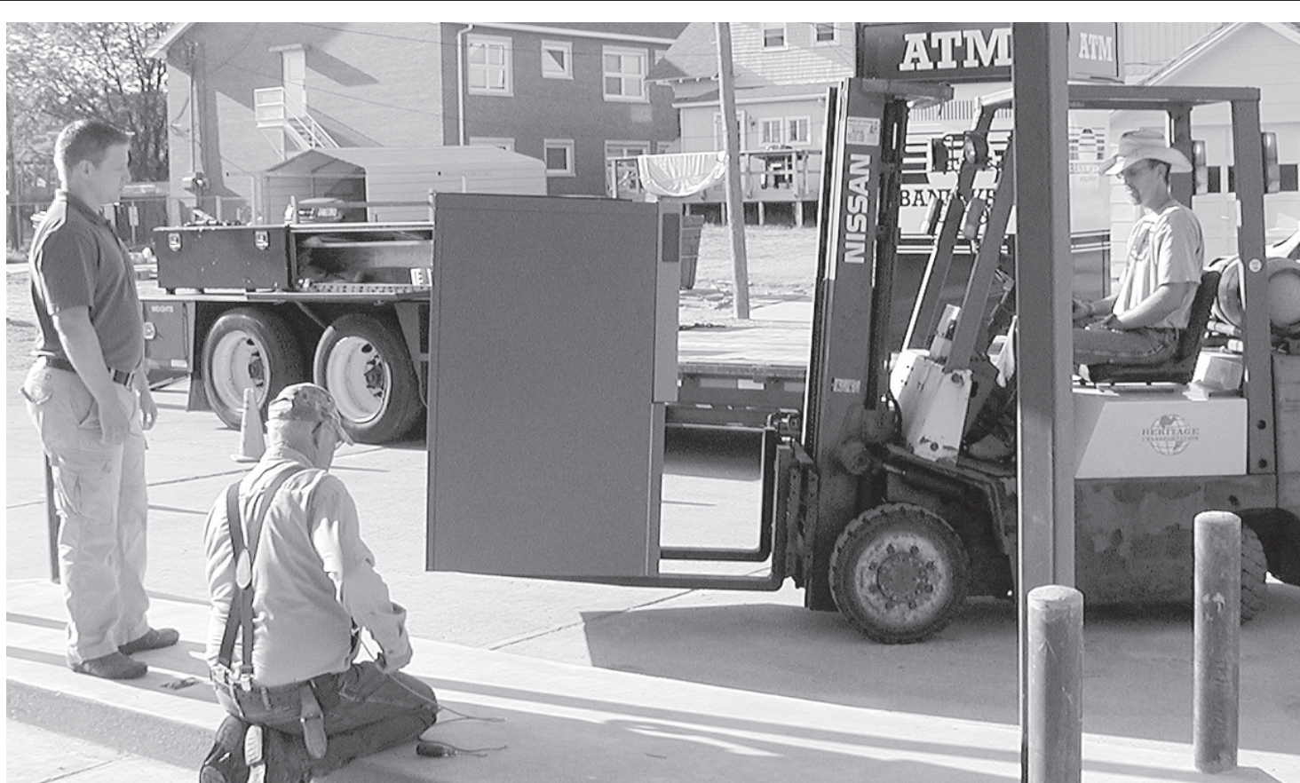
BANKWEST INSTALLED a new ATM machine on the south side of bank. Workers were busy getting the equipment set on Wednesday morning. There is also new curb and gutter. Herald staff photo by Casey McCormick
