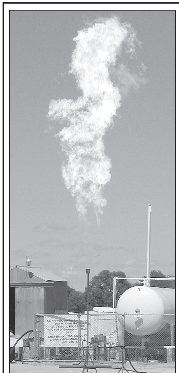
BURNING OFF THE VAPOR PRESSURE — Kevin Kowalczyk with Tedmon Welding was burning off the vapor pressures in the Equity propane tanks Tuesday. New valves will be installed bringing the tanks up to regulations. Herald staff photo by Karen Krien
