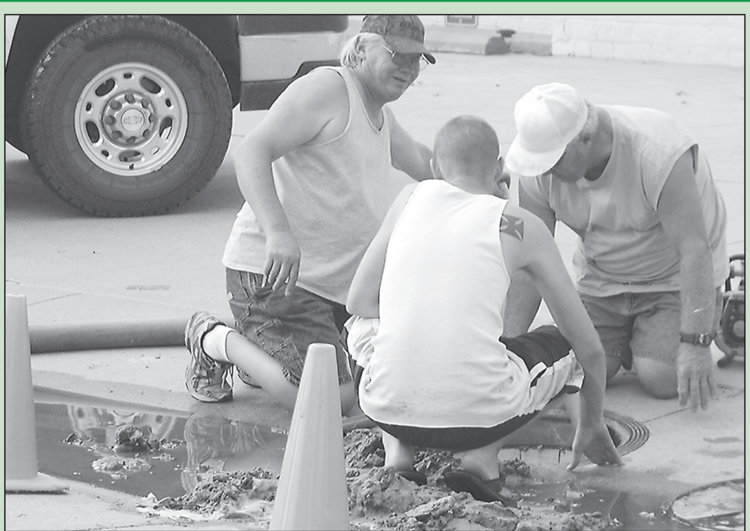
IT ISN'T WINTER! Instead the temperatures were in the high 90s when the St. Francis city crew was called to fix a broken water meter on Main Street Sunday afternoon. The water was flowing out the meter hole onto the street when they arrived. Generally, water meters break when it is freezing. Pictured are John Larson, Paul Larson and Glenn Schliep. Herald staff photo by Karen Krien
