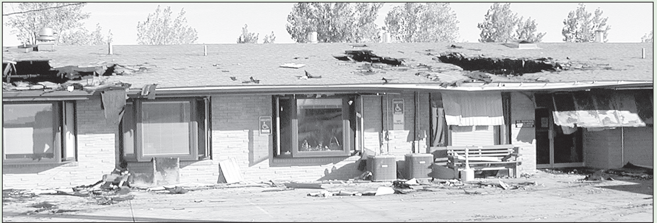
THE DAY AFTER THE FIRE, much of the damage on the south side of the Good Samaritan Village could be seen.
