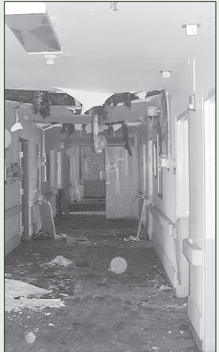
AFTER THE FIRE, this photo showed some of the damage to the hallway at the Village.
