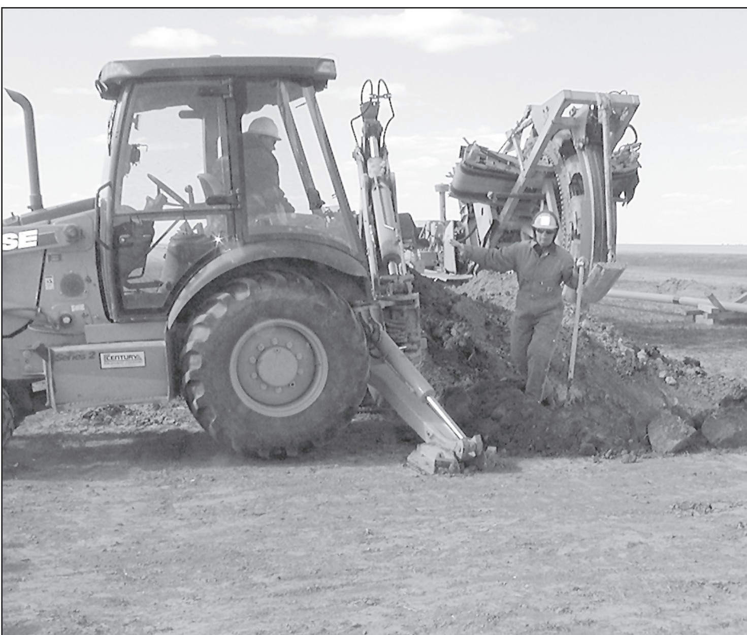
LAYING A PIPELINE , Lester Baker and Joyce McArthur from Wray, Colo., were working on the 21 mile gas line. It runs along Highway 36 from Bird City to east of St. Francis. Herald staff photo by Norma Martinez.
