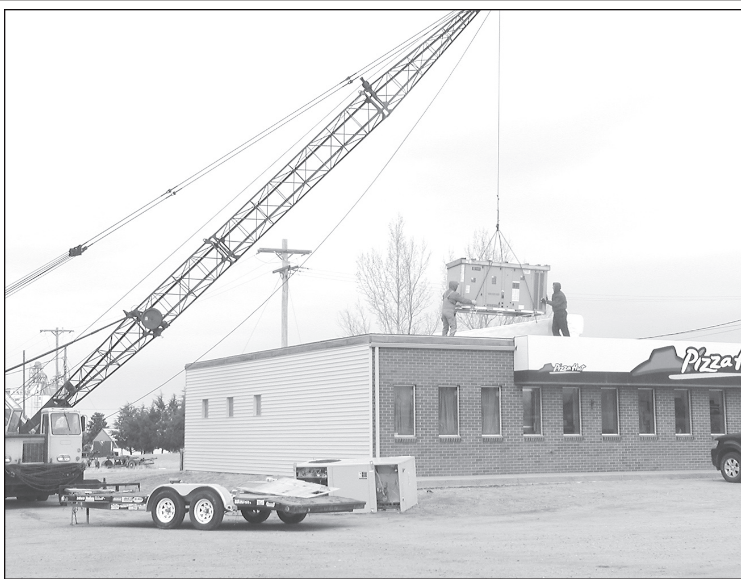
AFTER THREE WEEKS, the Pizza Hut had a new furnace installed on the roof of the building. Ed Marin and Kurt Bucholtz, Lampe Hardware, were on the roof as the county crane lifted the huge furnace to the top.
