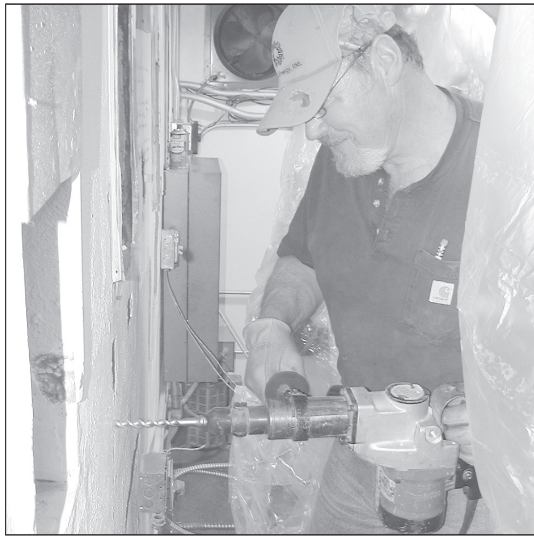
ROGER JENSEN drills a hole in the wall to install the new digital equipment at the theater. The wall is 14" thick.
