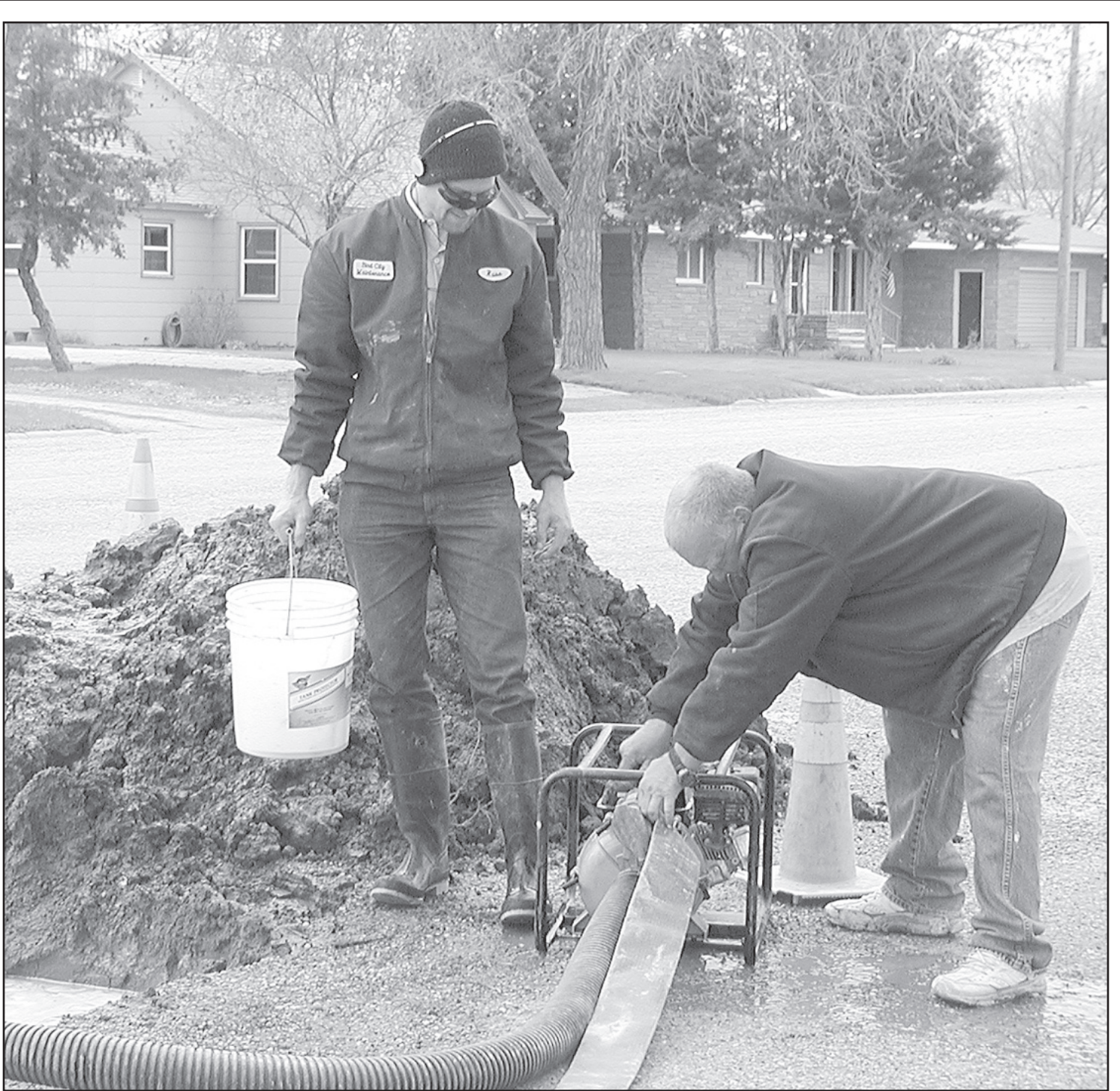
DRAINING A NEW LEAK on Bird Avenue is Russell Jackson, new maintenance employee and Brad Schneider. The city has had two leaks since the weather is warming up. City Council has hired a company to measure water usage and determine the areas where the pumps are losing water. Mr. Miller is also looking into funding for replacing water systems.
