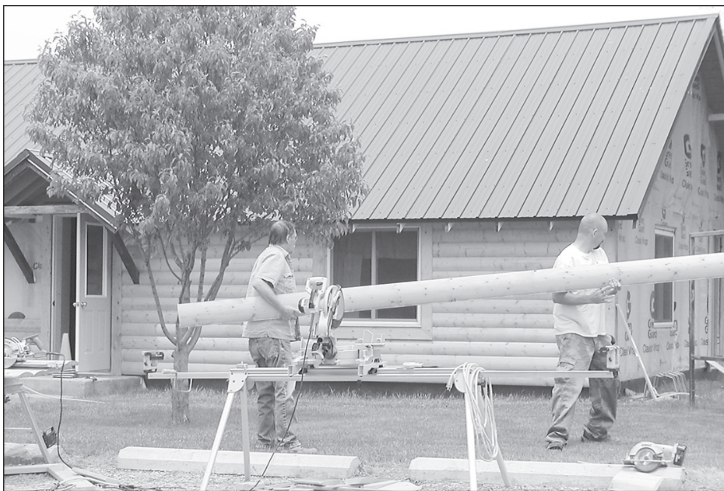
GARDNER CONSTRUCTION got the bid to side the Scout Hut. Getting ready to put up another piece of log siding is Chet Gardner and owner, Justin Gardner.
